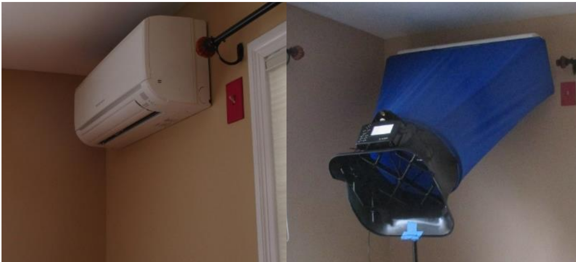
Figure 3. DHP Supply Airflow Spot Measurement
