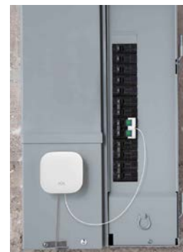
EMF sensor installed at breaker panel
