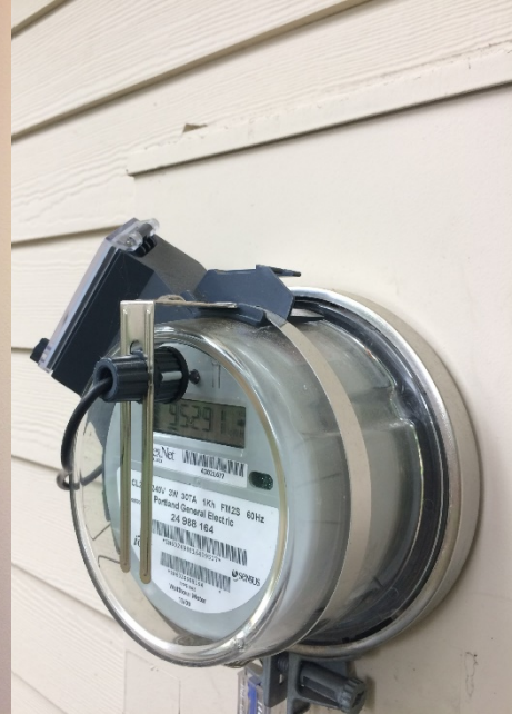
Attached to Utility Meter
