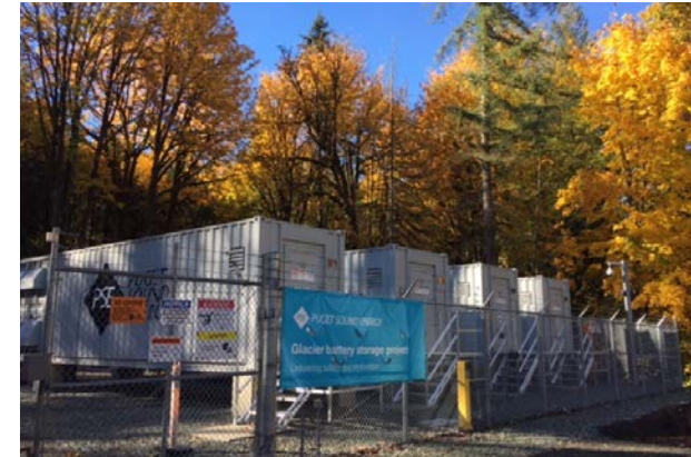
Glacier Battery Storage Project
